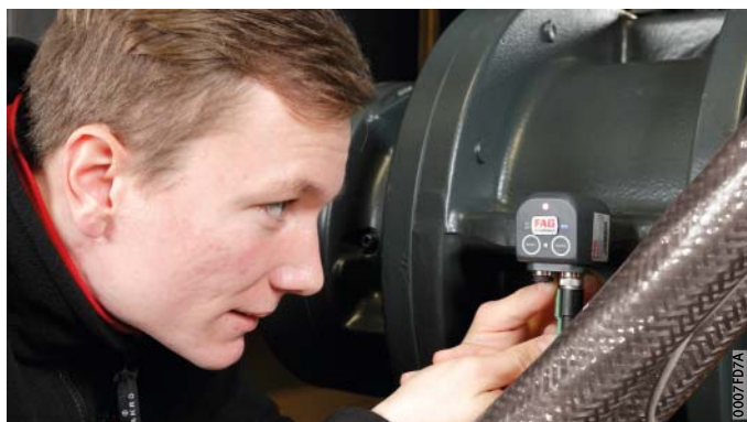
Figure 3 Commissioning of FAG SmartCheck
